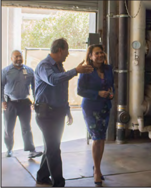
Roberto Valadez, Director of Engineering, leads Congresswoman Veronica Escobar on a tour through the UMC power plant.
